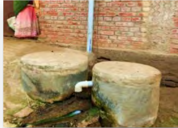
Defective Septic Tank & Soak pit
