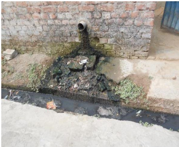
Black water from Septic tank
