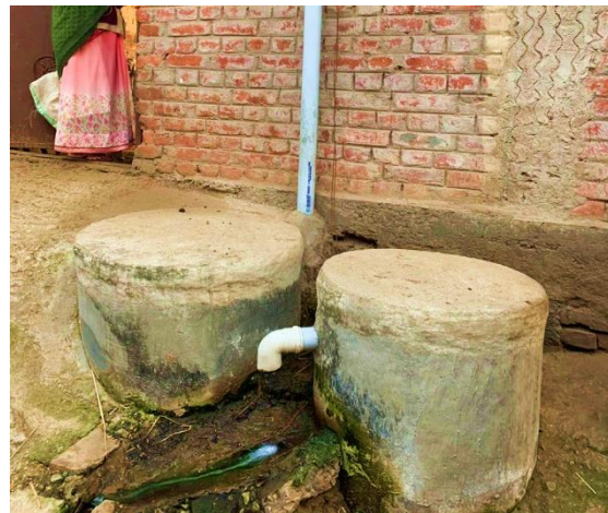
Black water from Single pit
